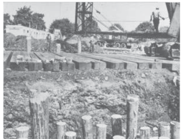
Foundation work is underway for the New York State Pavilion Progress Report #6, September 12, 1962
